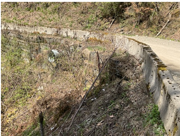
Outlet and some bulging wwm facing
