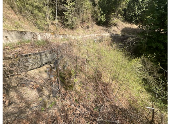
Geofabric at woods side has no wwm re enforcement and is failing.
