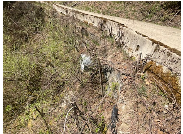
Foundation looks ok but erodible material. Sagging facing indicates this.
